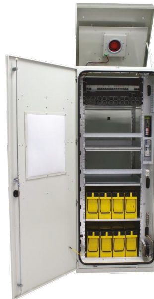
40RU enclosure with DFC cooling and 5RU Guardian power system
