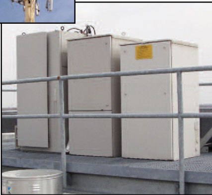
Typical Wireless Application
