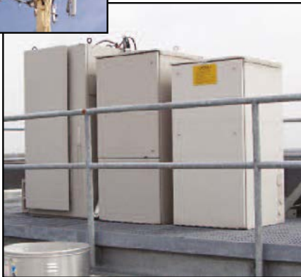
Typical Wireless Application
